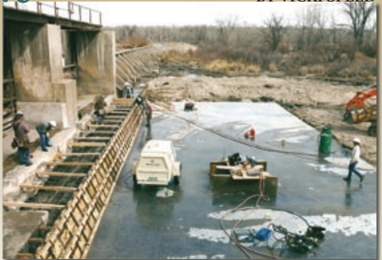
Diamondback Concrete Construction of Fort Morgan, Colo., does concrete work on projects of all sizes and types. Here the project is renovation and improvement of an aging concrete dam and its spillway.
