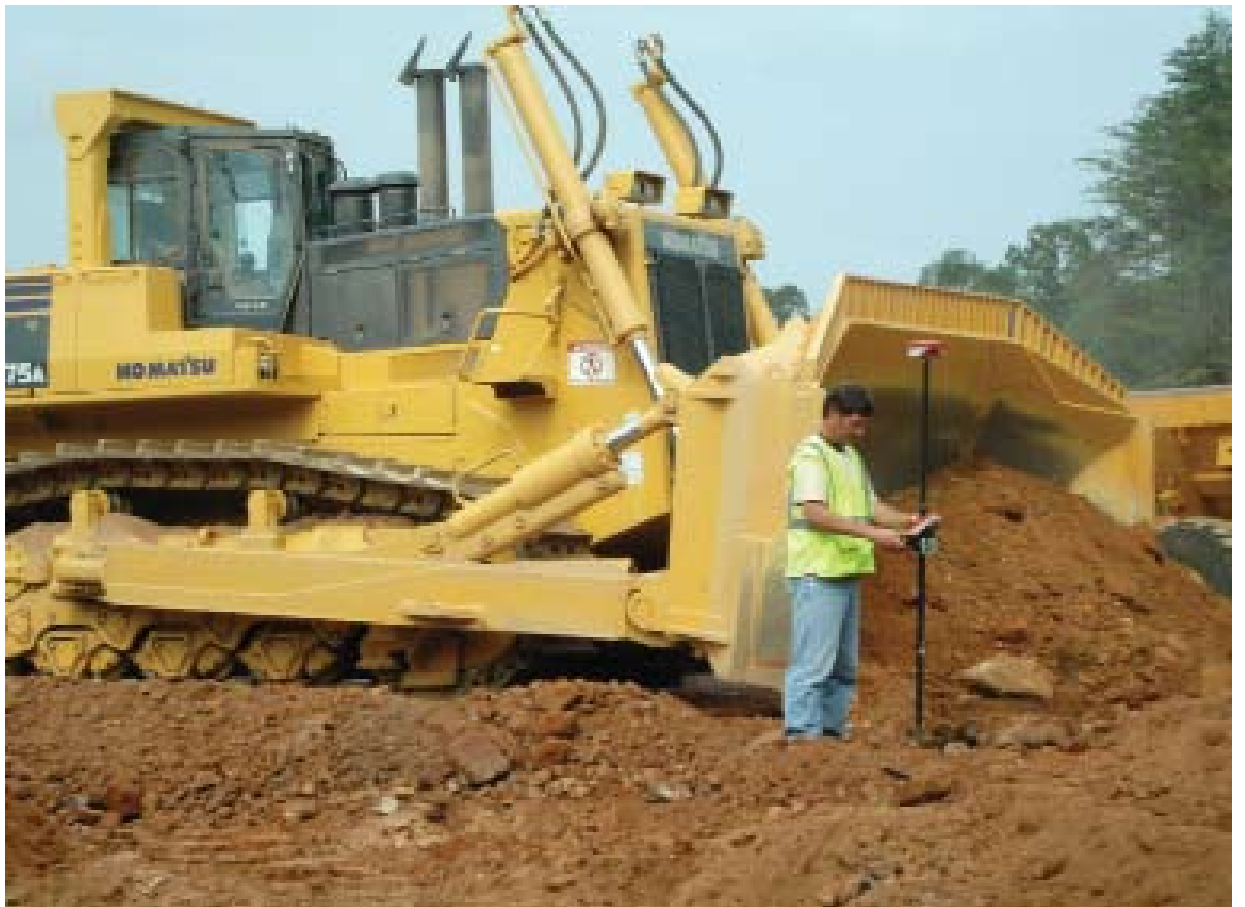
Ellis Astin Grading is using GPS-based technology to improve surveying and staking accuracy. The result has been greater productivity and efficiency on excavating and grading projects.
